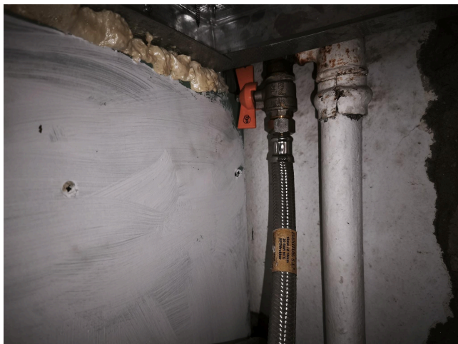
Cold water riser
