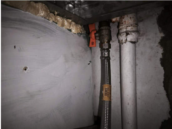
Water riser and main shutoff valve
