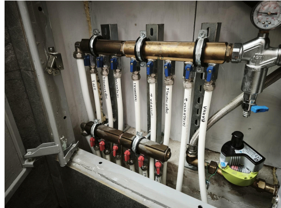
Water meter, cold&hot water manifolds in bathroom2
