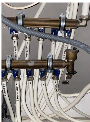
Heating system manifold
